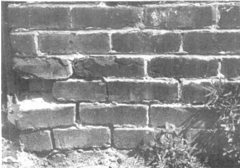
Water wicking up from the ground can rapidly deteriorate the first couple of feet of brick wall that's insulated on the interior—all for the lack of a capillary break in the brick.
