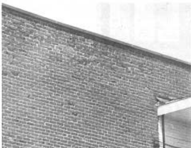
It's very common nowadays to see a band of deteriorated brick on the top of a house—usually about six inches above the newly insulated ceiling.
