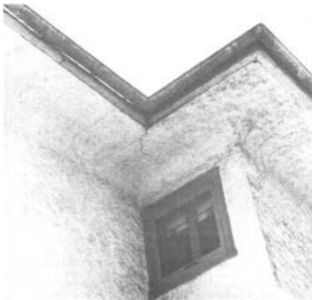
Points where roofs and walls meet are common problem spots. Cracks here may be one of the first signs of stucco damage to come.
