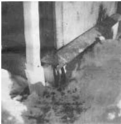
Frost heaving buckled the fiberglass facing on this basement insulation. The cure: non-frost-susceptible backfill, or switch to interior insulation.
