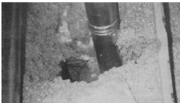
Figure 1. A chaseway for furnace and water-heater flues. The fiberglass batt used to block opening is streaked with dirt from leaking air.
