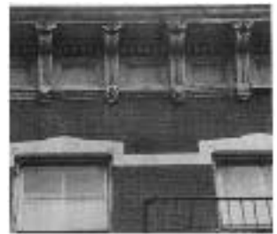
A glance from the ground indicates only minor problems with this cornice. A closer look reveals deflecting bricks in the parapet, and an unsound structural condition.
