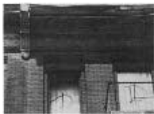
Deteriorated roofing and flashing have allowed water penetration into this cornice, rotting the interior supports. Parts have begun to pop off onto unsuspecting passersby.
