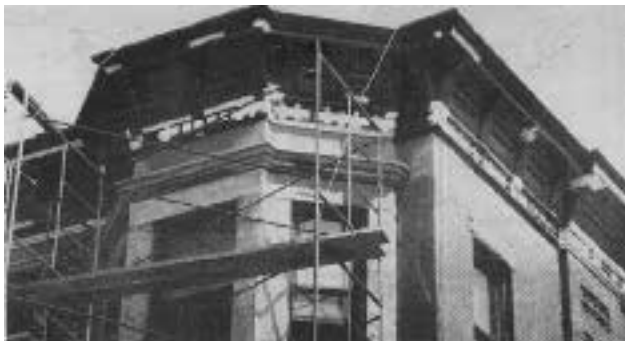
With few surfaces that would trap moisture, this cornice has held up well. White pieces indicate replaced parts. Samples of each have been saved for future reference.
