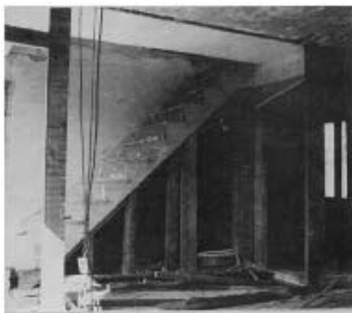
Water damage had totalled the building's interior when they found it (left). Restoration work (right) was faithful to the original and finely crafted, but not quite right for the market.
