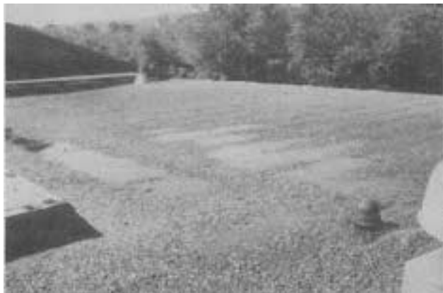
Damaged by winter condensation, the Tectum deck on this New Hampshire roof has sagged between the bar joists. Pounded water now collects in the depressed areas.
