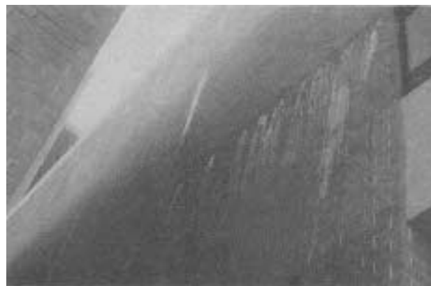
Ice on the walls of this hospital are a symptom of the multi-million dollar damage caused by a defective vapor barrier. The brick veneer, gypsum sheathing, and steel ties are all deteriorating from constant wetness.
