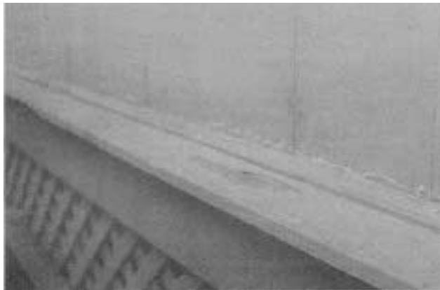
This shelf gets dripped on from the roof and sits in snow all winter. These are tough conditions for even the best paint job.
