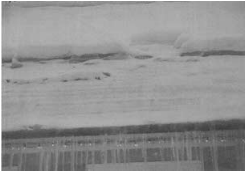
Keeping the lower portion of the roof clean with a shovel or snow rake only shifts the ice dam farther up the roof to the bottom of the snow blanket.
