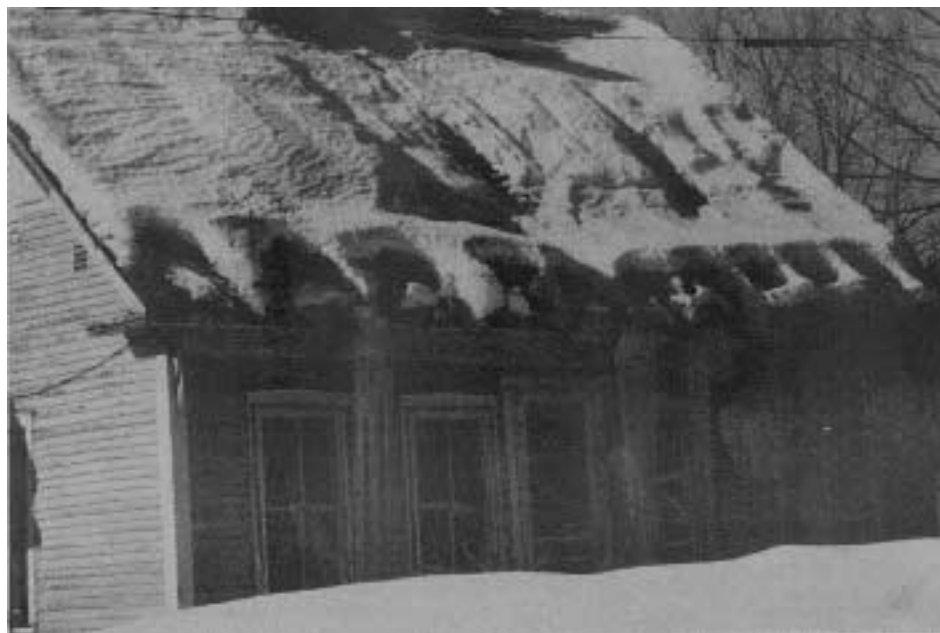
Electric cables do not prevent ice dams — they merely change their shape into a distinctive zigzag pattern.
