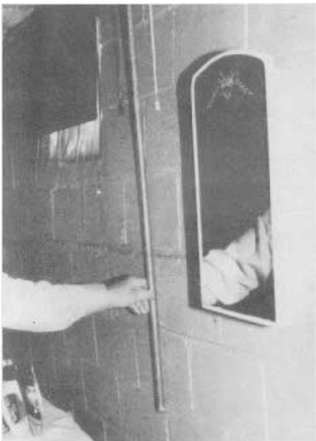
Check the amount of bowing with a straightedge. If the amount of deflection is one-third the thickness of the wall, then part of the wall is in tension, and the wall will be structurally unstable.
