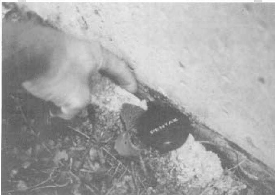
During dry spells, expansive clay soils shrink and pull away from the foundation wall.
