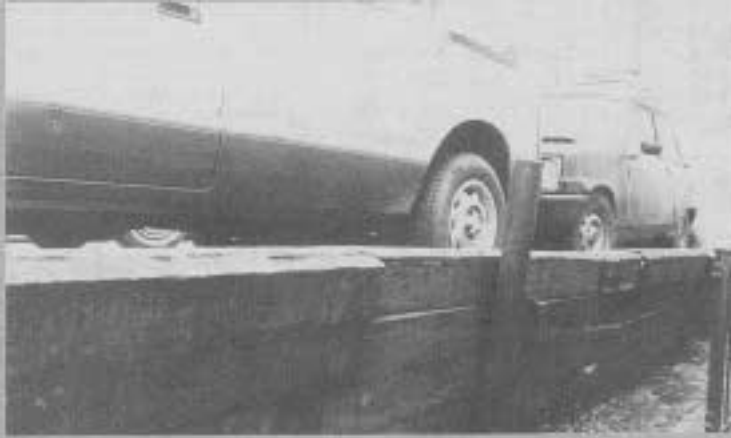
This timber crib wall (top) leans dangerously under the surcharge from the autos above. More timbers tied into the upper slope might have helped. A similar structure (bottom) uses concrete "logs" to successfully form earth-holding cribs.
