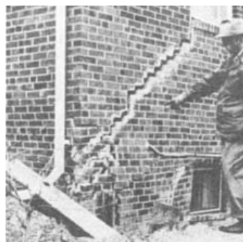
Soil with a high clay content often swells when wet and shrinks when dry. This difference in volume between wet and dry conditions — up to 50% — can cause damage like this.
