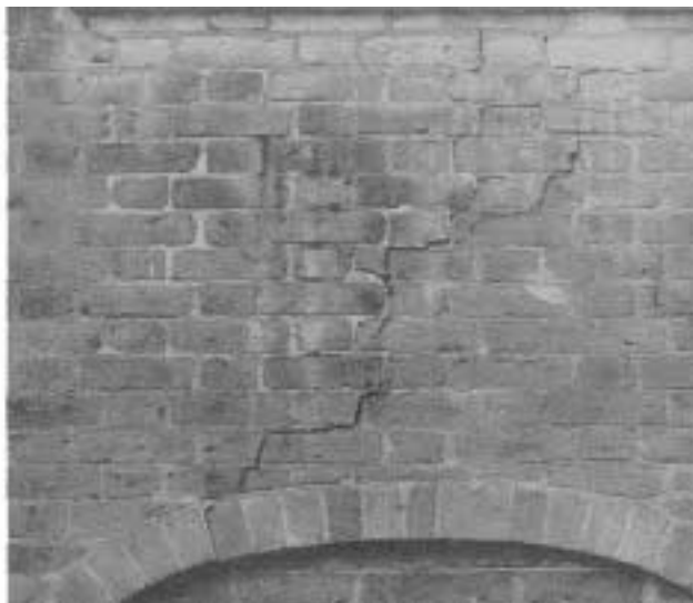
Any structural cracks must be analyzed and repaired, if needed, prior to repointing. Such cracks are common near windows and arches.
