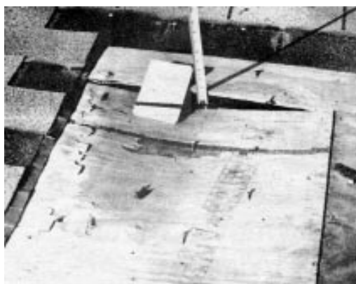
A 1 3/4-inch deflection of this FRT roof sheathing causes a cracking over the truss, left.
