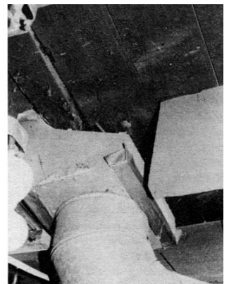
Figure 5. The joist was in his way, so the sheet metal worker cut it off. Alternative support is now needed.
