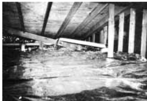
Figure 4. The findings are inconsistent, but current research indicates that dust will impair the performance of attic-floor installations. Attic access could also be a problem.
