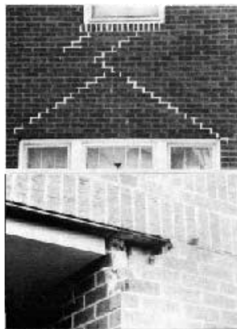
Figure 5. Deflection of a wood window frame caused the triangular chunk of brick above the window to drop. The brick was only supported by the window frame.
