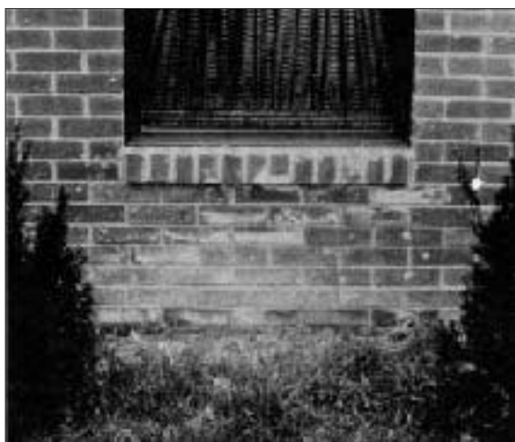
Figure A. White powder on the surface of masonry indicates the brick is saturated with water.
