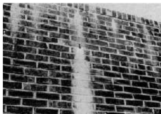
Figure D. Water spilling out weep holes leaves a trail of efflorescence. With no flashing to cover the flat brick parapet ledge, damage like this is bound to happen.
