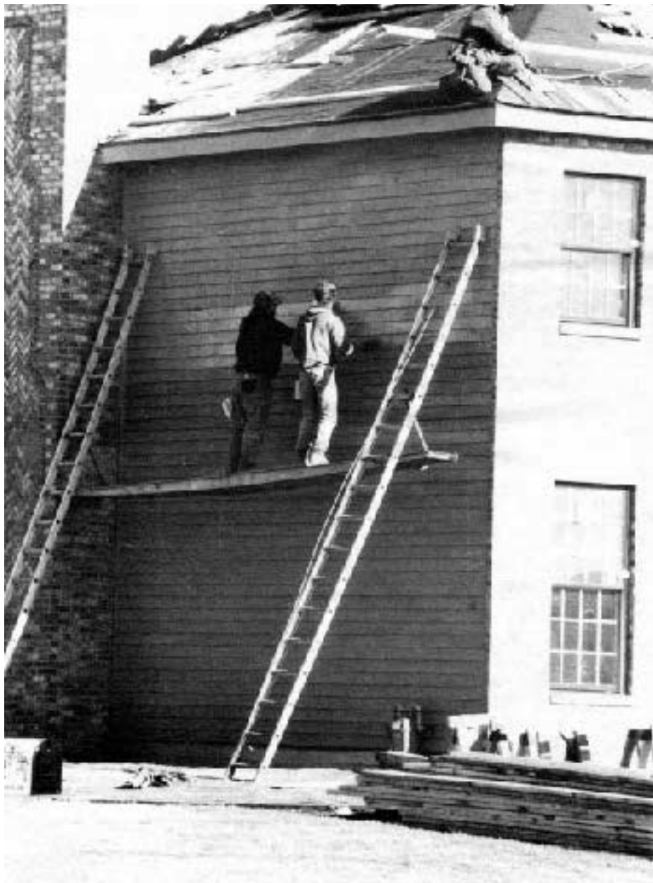
The two guys working off the ladders are using a safe OSHA-approved set-up. The roofer, on the other hand, should have roof brackets and a safety line.
