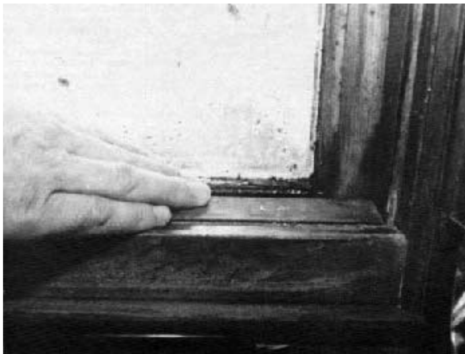
When windows show this much condensation, humidity levels are too high and should be corrected by eliminating moisture sources and increasing ventilation.
