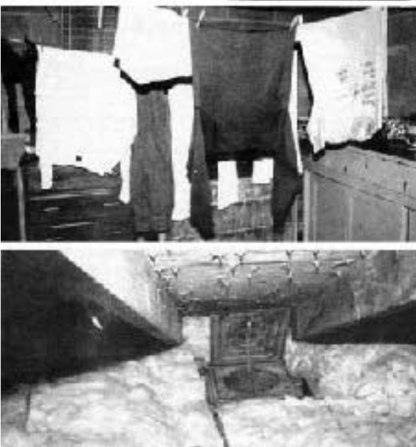
Figure 6. These sources of excess moisture—a shower without an exhaust fan, clothes drying in the basement, and a bathroom exhaust vented into the attic—are easy to fix if homeowner and builder are aware of the damage they can cause.
