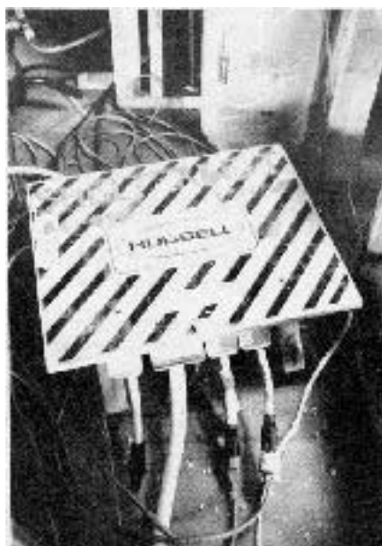
Figure 4. A fixture on large commercial jobs, 220-volt spider boxes bring 100-volt and 220-volt receptacles right to the center of the job. This allows shorter runs of smaller-gauge drop cords, and keeps connections at the power pole to a minimum.
