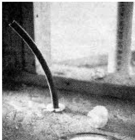
Figure 3. A plastic insulator protects this polybutylene supply line from damage by the subfloor sheathing. The toilet supply line will get an additional shut-off valve at the fixture before final hookup.
