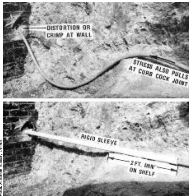
Figure 2. In many PB water-service systems, piping has been damaged due to earth settlement (top). Problems include shearing of the tubing at the foundation wall. To prevent such failures, model codes recommend you use a rigid PVC sleeve from the foundation across the footing trench and onto undisturbed soil for a distance of 2 feet (bottom).
