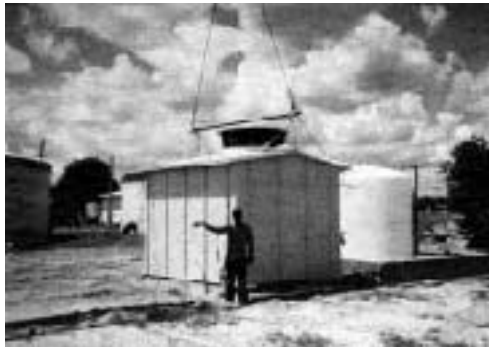
Figure 2. Pultruded plastics are strong but costly. They are used primarily for special construction needs such as these all-plastic outbuildings used in pulp mills and other corrosive environments.
