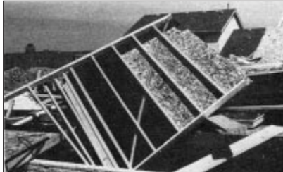
Figure 2. Shear-wall sheathing and a diagonal T-brace held some walls together, but they still pulled away from the platform.
