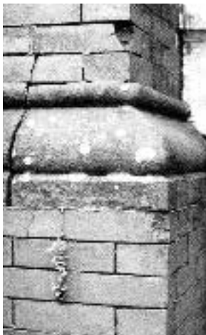
Figure 2. The brick below the stone can be repointed, but the masonry above needs structural work since the bricks have cracked.
