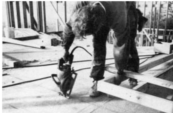
Figure 2. Production framing crews prefer worm-drive saws because much of the cutting is done in place rather than on benches or horses. Dunkley requires his crew to bring their own saws, but backs those up with three Skil Model 77s of his own.
