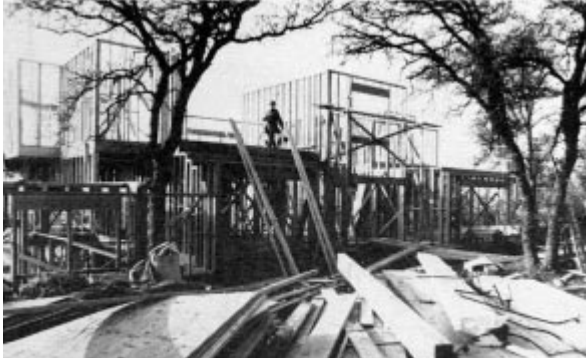
Figure 1. Houses we frame are rarely on flat lots, and often exceed 3,200 square feet. This one has a two-story curved entry, 18-foot walls in open areas and lots of roof complications.
