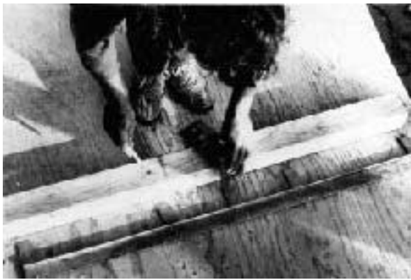
Figure 4. These two production tools—an aluminum layout stick and a chisel marker—can easily be fabricated onsite, or with a little sheet metal in the shop. The layout stick is used to quickly mark 16-inch and 24-inch centers; a chisel marker can scribe partition or corner intersections of 2x4 or 2x6 wall.
