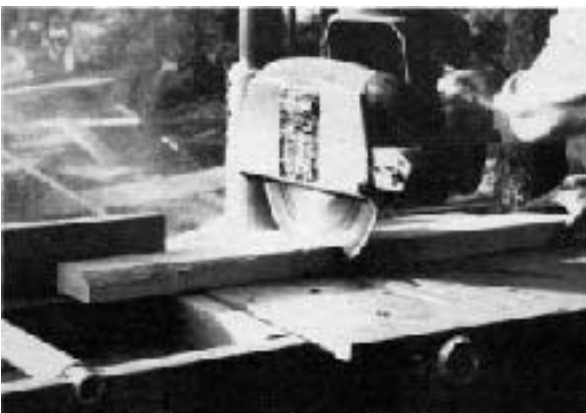
Figure 3. A Delta 12-inch radial-arm saw makes the trip to the job site every morning, but the site-built outfeed tables and saw stand stay put. The rollers are lengths of 1 1/4-inch PVC pipe that spin freely on fixed lengths of 1-inch stock notched into the table rails.
