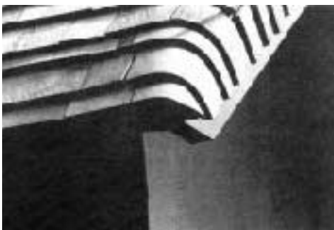
The curved shingles on the edges are perhaps the most conspicuous feature of this distinct roof. Some of the shingles near the bottom of the picture are bent a full 90 degrees around the corner.
