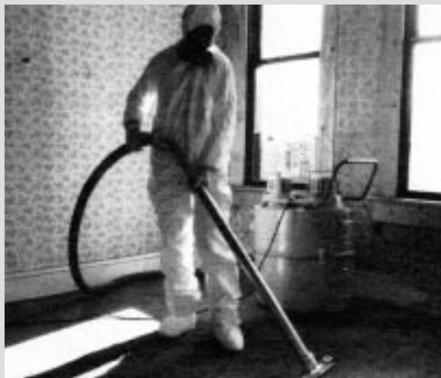
Current HUD lead paint abatement methods require specialized training and protective clothing.
