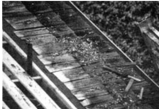
When roofers investigated woodpecker damage to the wood shingles on this California condo project, they found thousands of acorns stuffed under the sheathing.
