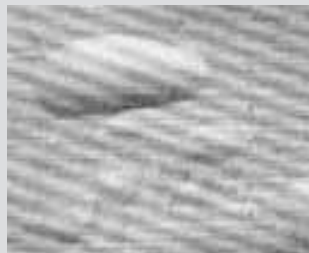
Blistering paint is the unsightly result of moisture pushing through from the interior of the building. Backpriming the siding is the preferred method of preventing the problem.
