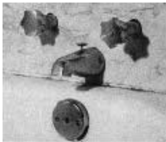
Water will penetrate the wall at the faucet handles (above) whenever the shower is used. The holes should have been covered with trim plates sealed with plumber's putty. The curling and torn linoleum around the toilet (right) indicates water damage to the underlayment, probably from a faulty toilet seal.
