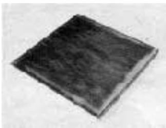
Wrong tile for the job: The glaze along one edge of this wall tile is worn completely through — because it was mistakenly installed on a floor.
