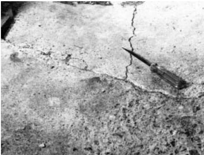
Bad substrates equal failed tile: Don't even think of tiling over a crumbling slab with structural cracks 1/8 inch or wider.
