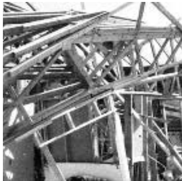
Poorly secured trusses and roof sheathing were the most common failures in the homes destroyed by Hurricane Andrew. Initial investigations suggest that shoddy construction, rather than inadequate codes, caused most of the building failures.
