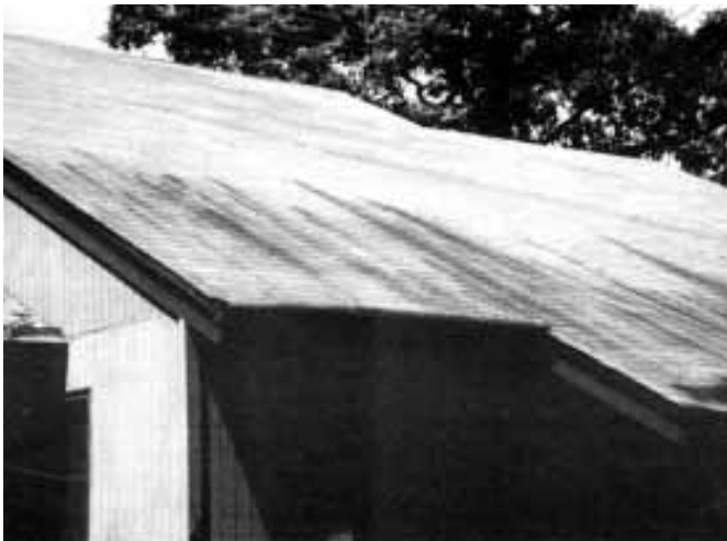
Black roof stains on this Virginia home are caused by a blue-green algae. The problem, which is common in warm, humid areas, can be avoided by using "fungus-resistant" shingles or by inserting small strips of zinc along the roof.
