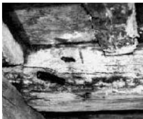
Figure 1. Dry, powdery surface decay extends 1/2 to 2 inches into the timbers. Half of the 4-inch blade of the ice pick easily penetrates wood softened by insect and fungal decay.
