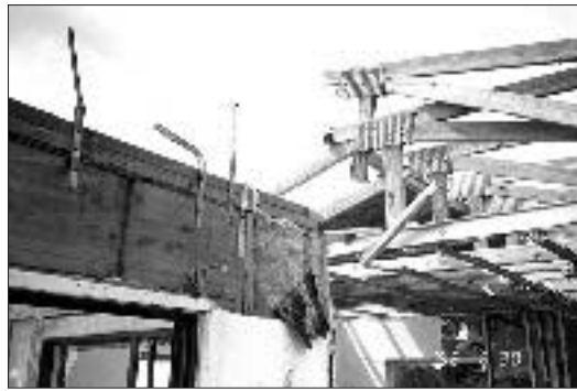
Figure 5. Not enough nails in these hurricane straps allowed the trusses to tear loose from the bearing wall they sat on. The straps must be nailed at every position on all sides of the truss, not just into the top edge.
