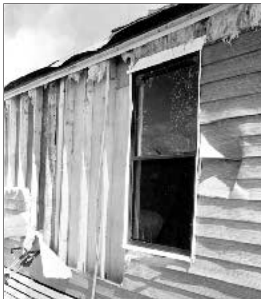
Figure 7. On wood-frame houses, stucco exteriors stood up much better than cladding such as hardboard and aluminum siding. These dented easily from debris and tore loose in many cases.
