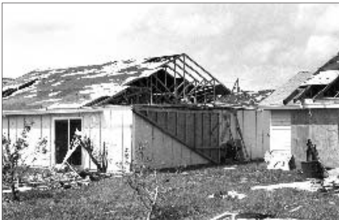
Figure 2. Countless wood-framed gable ends failed after the wind tore off the sheathing — a truss roof's primary lateral bracing. With the plywood gone, the joint between the wall and gable-end truss opened like a hinge.
