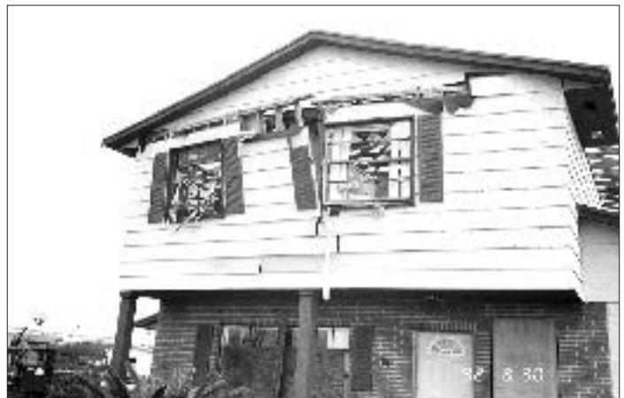
Figure 3. Some wood-framed gable ends failed, even with the roof sheathing intact, because of weak splices in the top plate above window openings.
