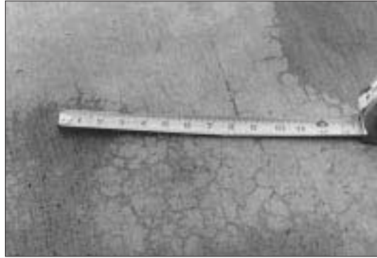
Figure 2. A visual defect called crazing results when moisture evaporates too quickly from fresh concrete.
