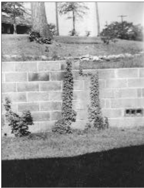
Figure 1. This block wall, which on its face looks sturdy and well-built, collapsed during heavy rains because it had no reinforcing, too small a footing, and was backfilled with native soil.
