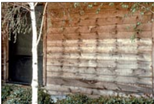
Figure 5. Rusting nails leave ugly streaks down the side of a building. The right nails are stainless steel or hot-dipped galvanized — not electrogalvanized.
