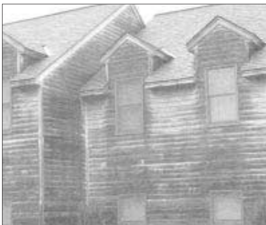
Figure 7. The silver-gray, weathered look that some clients desire happens naturally only where there's plenty of sunlight and salty air to discourage mildew growth. Left untreated, cedar siding is more likely to end up dark and blotchy.
