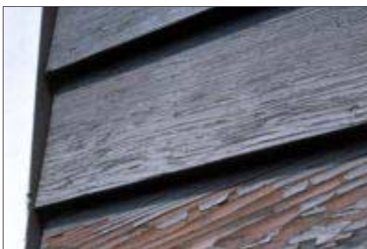
Figure 8. Solid-body stain applied directly to smooth siding has led to many failures. The solution: Use a primer first or put the rough side out. In either case, backbrush the finish if applied by spraying.
