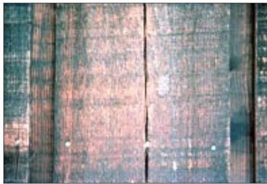
Figure 2. Nails at both edges and the middle of this wide piece of channel rustic (left) caused cracking. Two nails per board, 3 to 4 inches apart — with no nails through the overlap — is best. Bevel siding that is double-nailed is prone to cracking, particularly at the ends (below).
