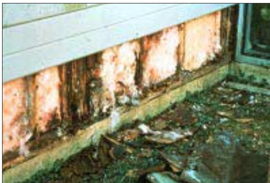
Figure 6. Siding is not waterproof. Here, water got into the wall cavity of a new home and rotted the studs and plates. Building paper would have prevented the problem.
