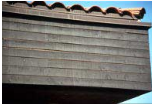
Figure 1. T&G is not a forgiving pattern. When installed green (left), it is bound to fail from excessive shrinkage. Even installed at 19% moisture content, the 1x10 siding (below) opened at numerous joints. A better choice would have been 1x6s, acclimatized for at least a week before installation.
