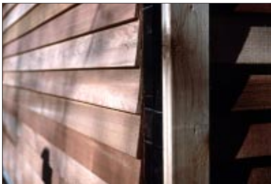
Figure 4. The carpenter nailed this bevel siding too high up, where the boards are thin and unsupported. This can cup and split the siding. The maximum overlap should be one inch.
