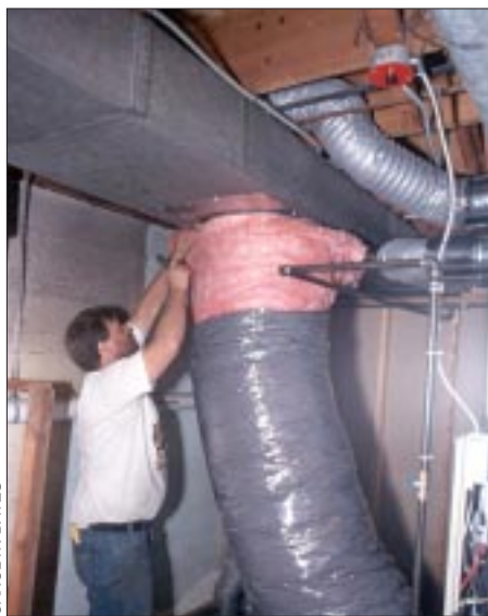
Figure 1. Using insulated duct on the return will dampen system noise, but you should oversize the duct to compensate for its higher resistance to air flow.
