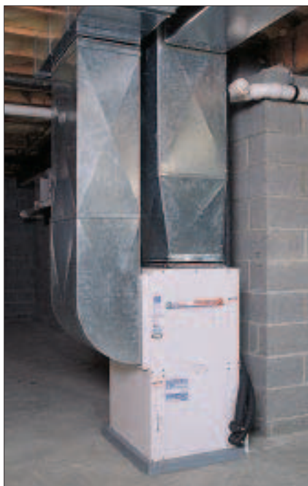
Figure 4. The heat pump unit is installed in the basement, where it is protected from the weather. Powered by house current, it does not produce combustion gases and does not need venting.
