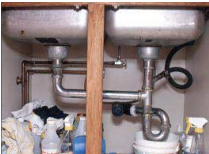
Figure A. A typical kitchen sink drain assembly, with its leak-prone slip fittings, leaves a lot to be desired. This two-sink setup has no less than six slip connections.
