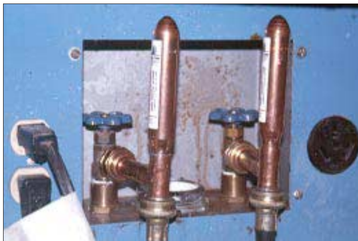
Figure K. Water hammer arrestors — not simply vertical pipes filled with air — are the best way to prevent water hammer.
