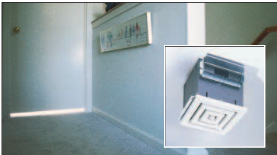
Figure 3. The Broan 360 Losone Ventilator provides exhaust for the author's ventilation system (inset). Undercutting interior passage doors helps ensure adequate airflow throughout the home, even when doors are shut (above).
