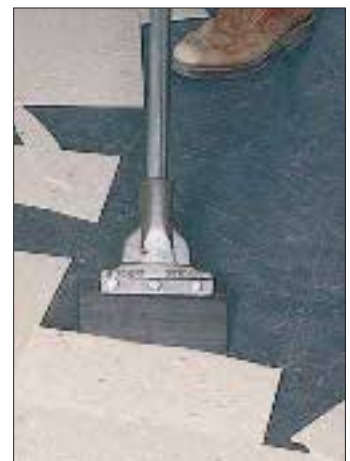
Under the new OSHA regulations, all pre-1980 floor tiles are assumed to contain asbestos unless tests prove otherwise.
