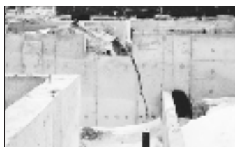
Liability claims for foundation failures like this can wipe out a small contractor's business.
