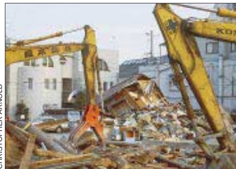
Many older Japanese homes were destroyed in the quake, but modern buildings nearby survived intact.
