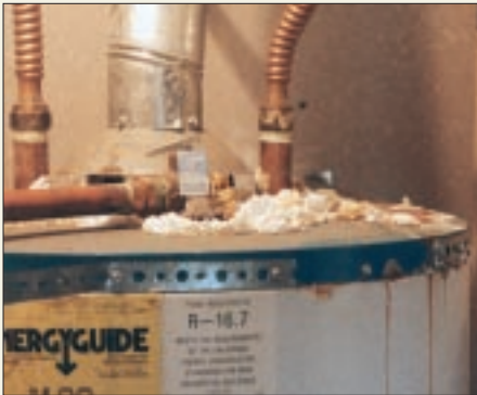
Figure A. Leaking at unions in the overhead plumbing caused this corrosion to accumulate on top of the water heater. Because the leaks went unnoticed for several years, repairs were made too late and the heater had to be replaced.
