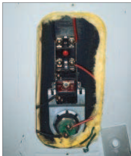
Figure 2. Lack of hot water from an electric water heater is often caused by a failed upper thermostat. Use a volt-ohm meter or pigtail tester to check for power at the two pairs of screws above and below the red reset button.
