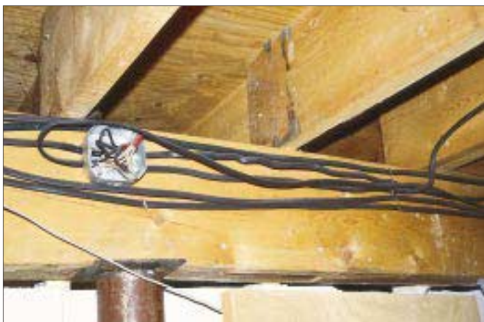
Figure 1. Sloppy wiring like this is an invitation to an inspector to check the job very carefully for further violations.
