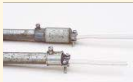
Figure B. When switching from one wiring method to another, code requires a changeover fitting (bottom) or a similar transition fitting made from standard parts (top).
