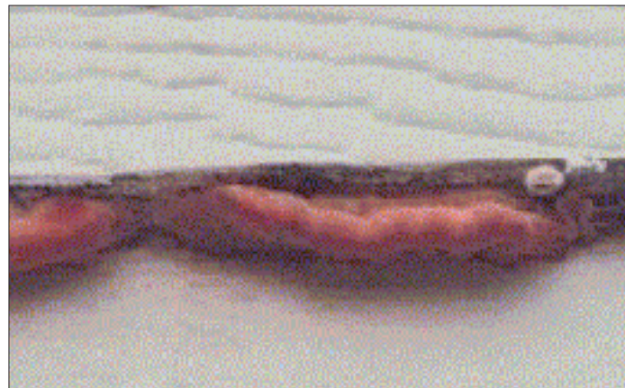
An image from Huntington Legal Advertising's World Wide Web page shows fungus growing from the underside of L-P Inner-Seal siding.
