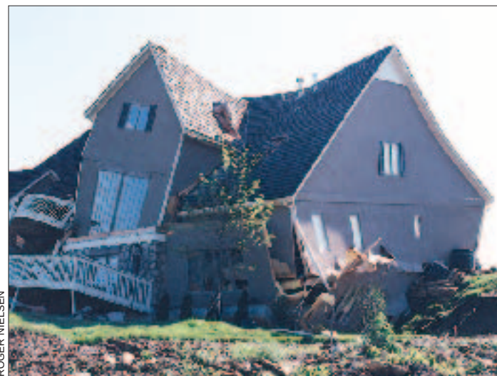
Shifting rock and soil caused the dramatic collapse of this new home in Overland Park, Kan.
