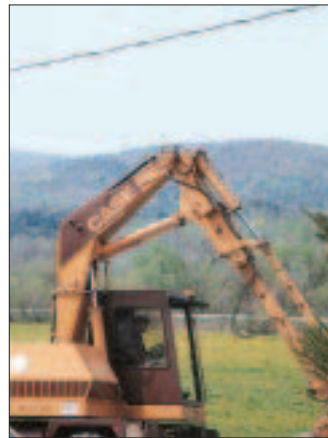
Boom trucks, cranes, and backhoes on the job pose an often unrecognized hazard. Contact with an overhead power line can be fatal.
